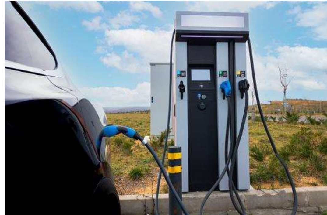
Electric vehicle charging station (example only)
